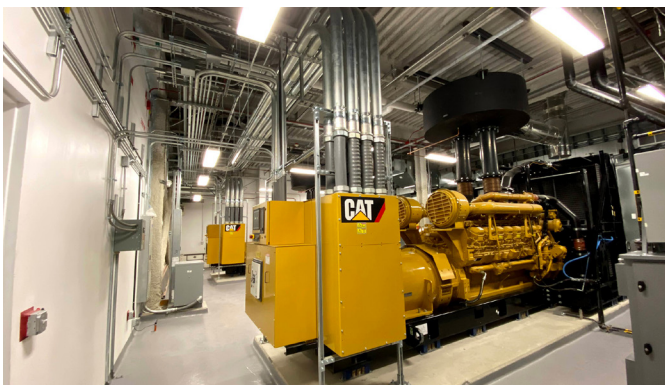
H Building Infrastructure Upgrades, Karpinski Engineering
