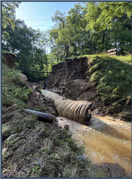
Palmer Township Culvert Washout
