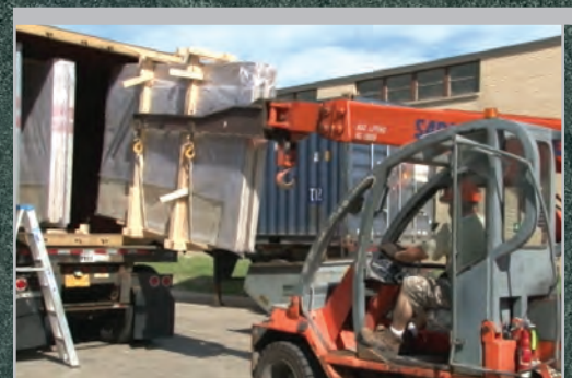
Mobile crane extracting a bundle from a container in an outside stone yard
