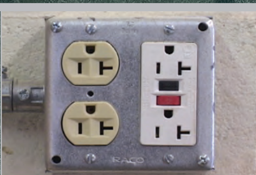
GFCI electrical outlet
