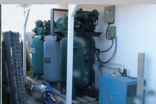
Compressed air tanks
