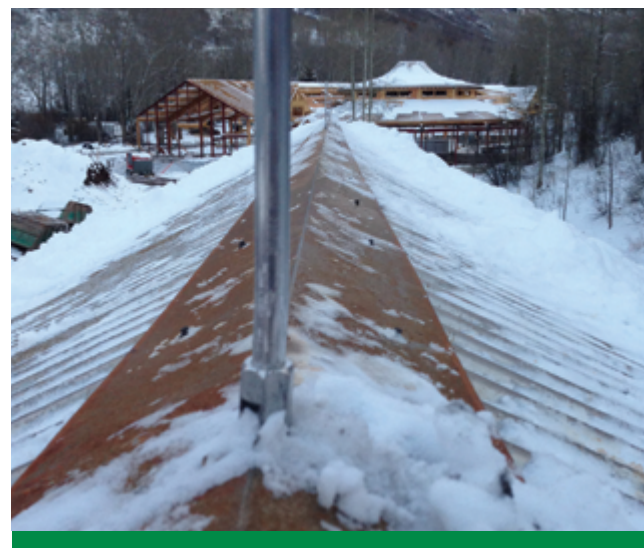
The air terminals on this ridge are supported from below the roof deck and sealed against weather intrusion. They are connected to each other and to ground by conductor cables inside the attic to maintain the design standards of this luxury resort development. Photo courtesy of Mr. Lightning.
