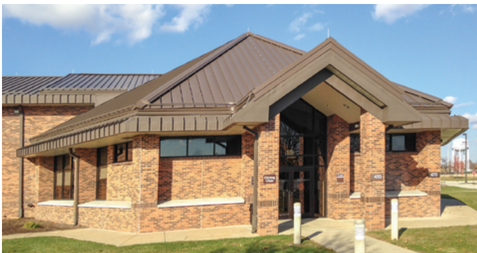
Air terminals must be located at high points and where indicated by NFPA 780. Conductor cables that are exposed to view should be installed along the natural lines of a building to minimize their visual impact. Photo courtesy of Guardian Equipment Company.
