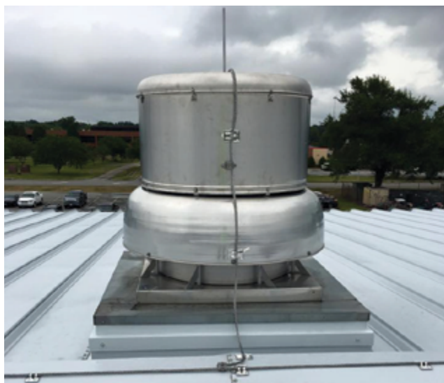
Air terminals must be installed on rooftop equipment that is not within the zone of protection created by air terminals mounted at a higher elevation on the building. Photo courtesy of Labeled Lightning Protection Inc.
