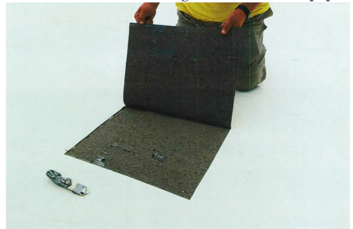
Figure 1. Moisture build up from concrete deck resulted in delamination of paper facer on polyiso board
