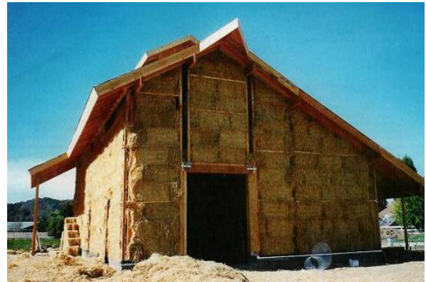
Figure 1-56. Non-structural straw bale walls prior to plastering. Image from the American Society of Agricultural and Biological Engineers. Used with permission.
