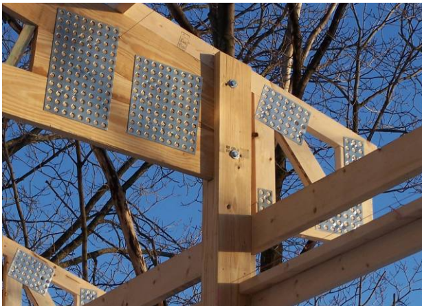
Figure 1-55. When truss is sandwiched between outer plies of a mechlam post, bolts are placed in double-shear for a very effective connection.
