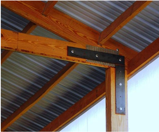
Figure 1-54. Truss resting on outer ply of a laminated post. Steel L-bracket placed on outer face of truss to help reinforce post-to-truss connection.
