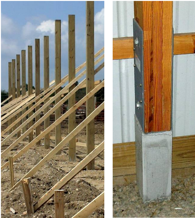
Figure 1-41. Preservative-treated, mechanically-laminated embedded post (left) and mechanically-laminated post attached to a precast concrete pier (right).
