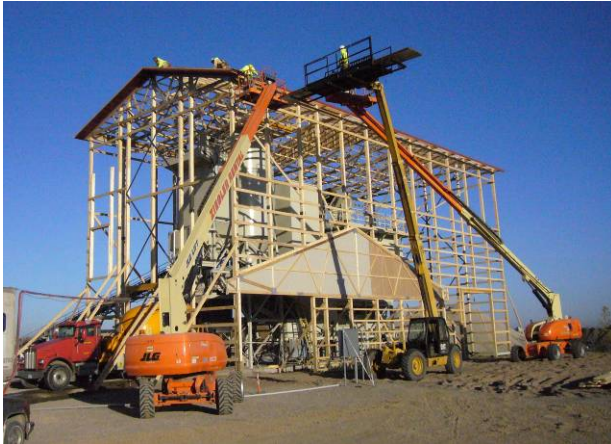
Figure 1-42. Post-frame concrete batch plant with a 45 ft ceiling height, accomplished in part by bracing wood columns back to the main structure of the concrete plant equipment.
