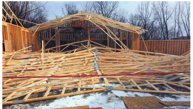
Figure 9. Progressive roof collapses during construction are due to the lack of temporary diagonal bracing on top chord CLR. The bottom image is of a conventional stick-frame building with 2-foot on-center trusses.
