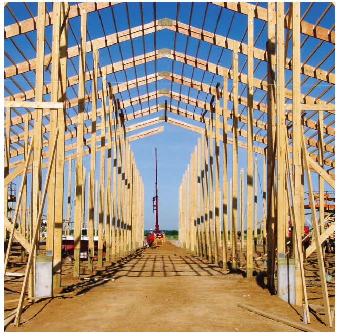
Figure 12. The lengthy interior posts being installed in this photo were five-ply glulam assemblies that did not require CLR to withstand design loads.
