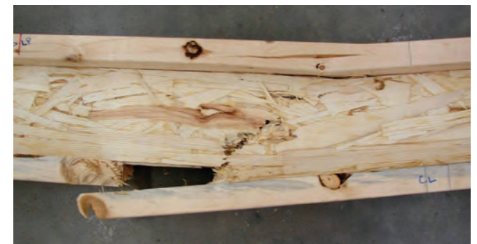
Figure 10. Typical I-AS failure through a knot in the tension flange near midspan.
