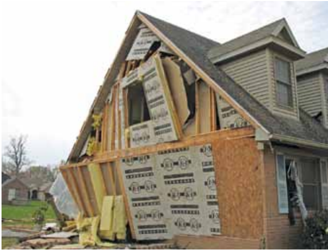
Figure 7 — Foam and vinyl wall covering failure. Note: the corner bracing was not what failed.
