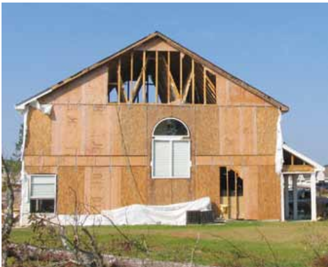
Figure 3 — Siding and non-structural sheathing wall covering failure. Rain following the wind event caused massive interior damage to interior finishes and personal property.
