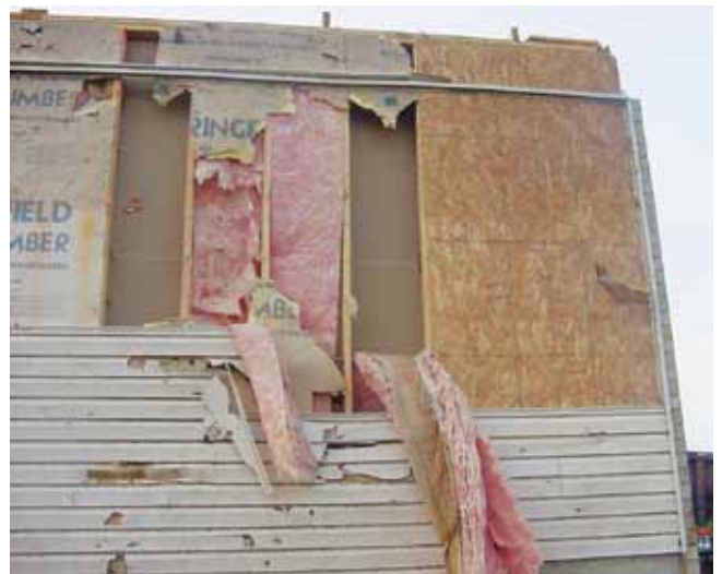
Figure 6 — Difference between structural and non-structural wall sheathing. Wind pressures act on all exterior surfaces, not just the corner bracing.
