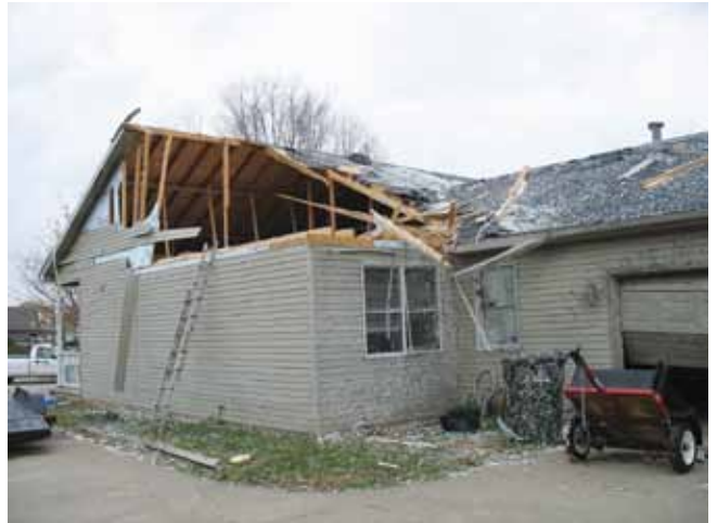
Figure 4 — Foam and vinyl wall covering failure. Note the roof damage caused when the breach in the gable-end wall pressurized the attic area.
