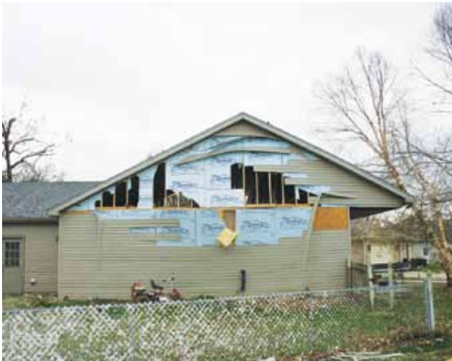
Figure 2 —Foam and vinyl wall covering failure.
