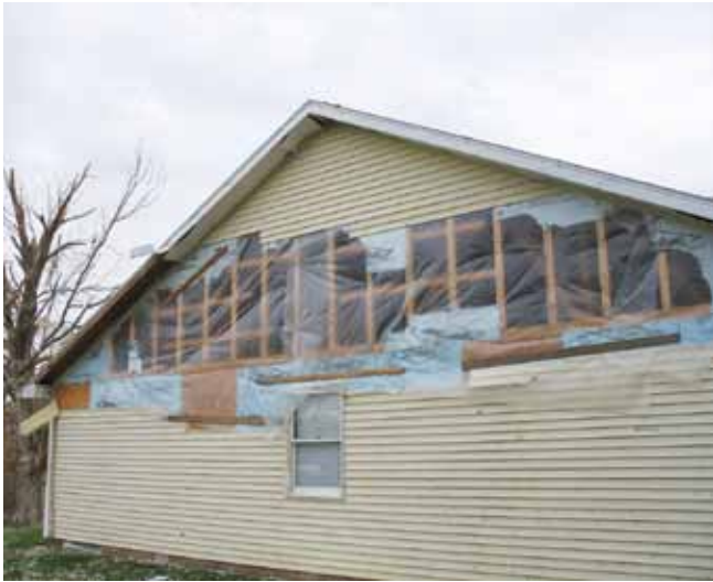
Figure 1 — Foam and vinyl wall covering failure.
