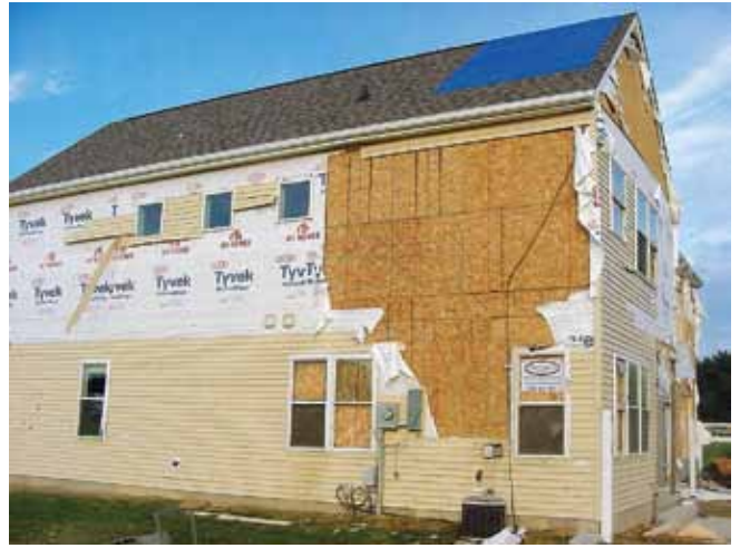
Figure 8 — Homes sheathed with continuous structural sheathing have significantly stronger resistance to the effects of wind pressures.
