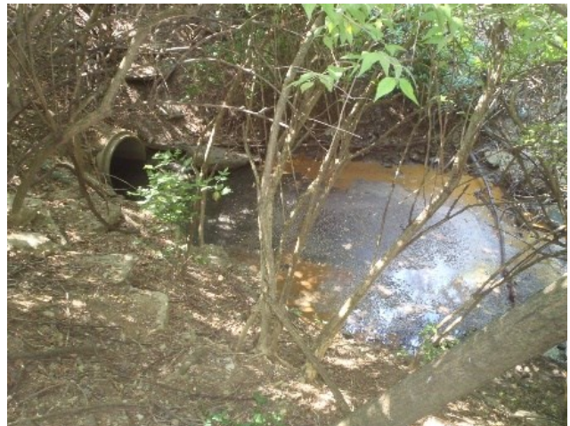
Figure 1: Contaminated water at outfall (July, 2012)
