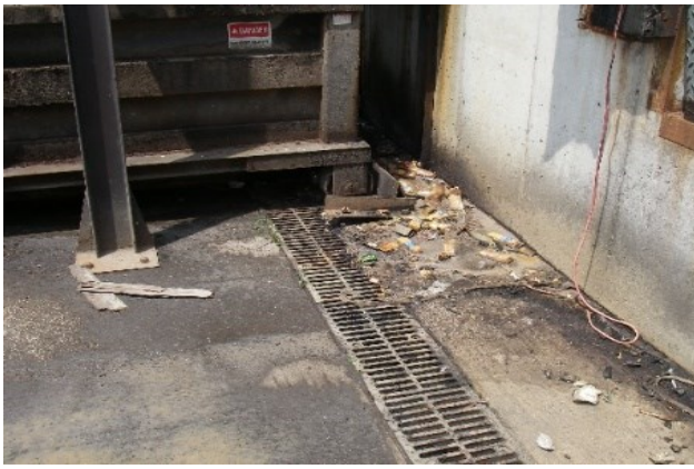
Figure 3: Garbage and leaking dumpster at trench drain (August, 2014)
